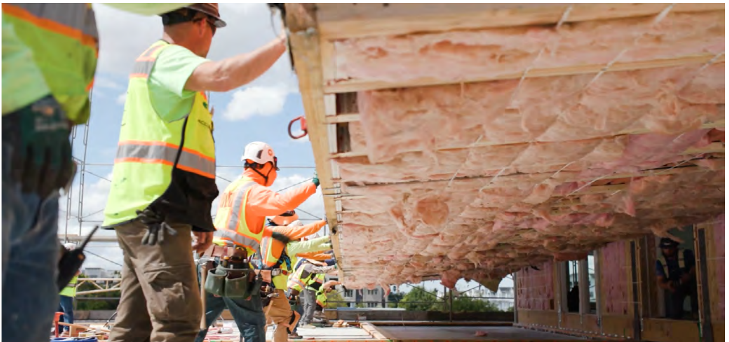
The Sango Court building was assembled over a 12-day period thanks to careful planning and expert consulting.
