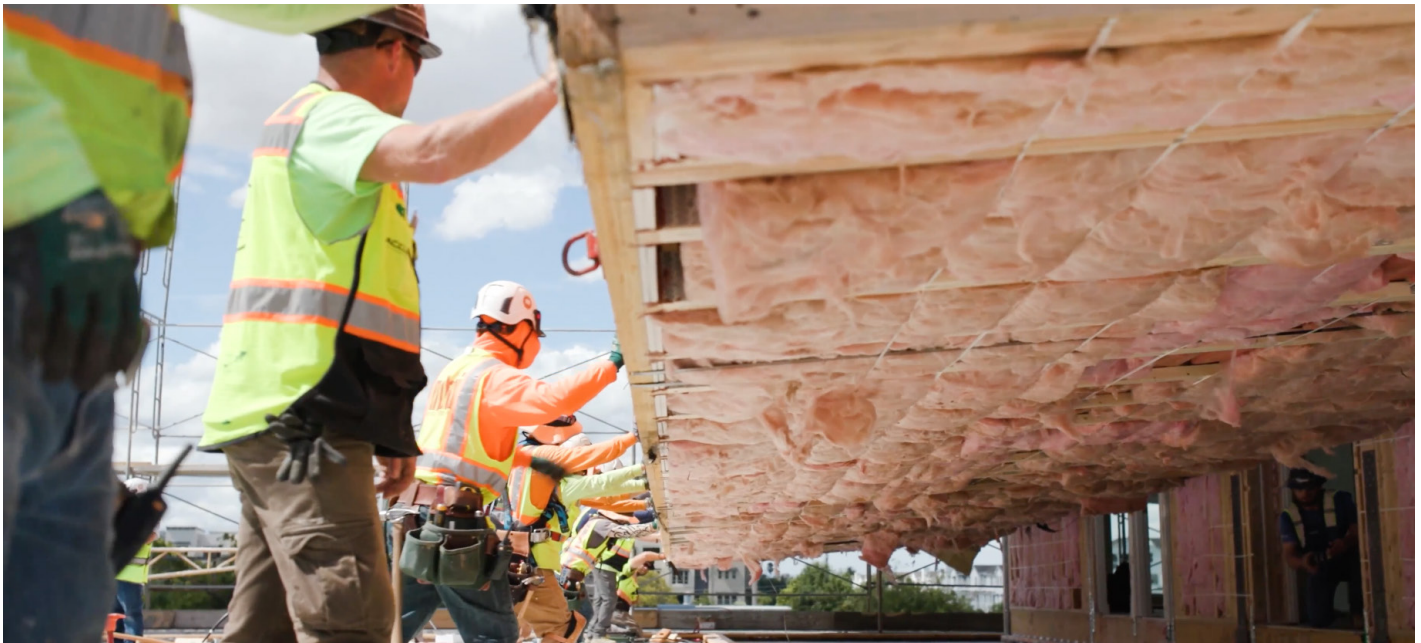
The Sango Court building was assembled over a 12-day period thanks to careful planning and expert consulting.
